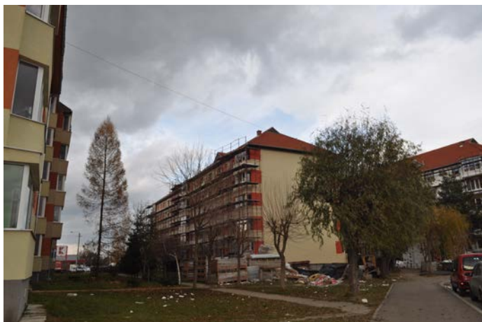
Picture 3 Littering problems trough delayed refurbishment
